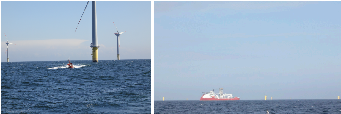
Image C05: Left) Dinghy for diving within alpha ventus . Divers checking, lying-up and obtain measuring instruments in test district alpha ventus . Right) Construction boat for offshore wind farm mounting close to alpha ventus .
