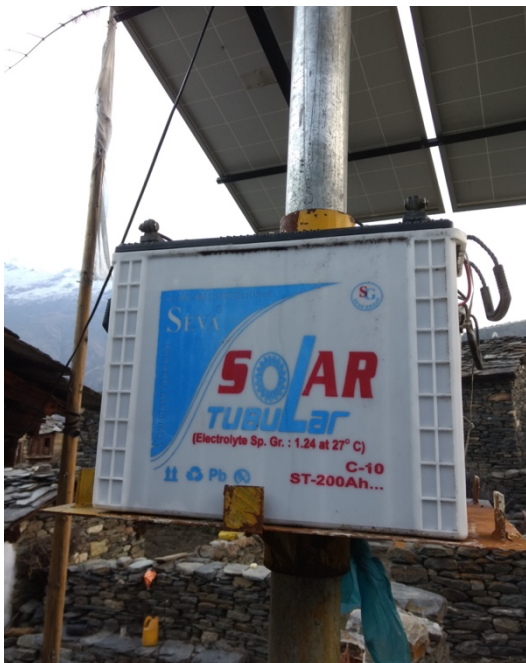
Figure 26 Solar powered streetlamps are seen in all villages in the valley
