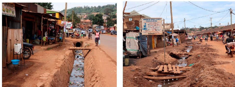
Figure 1. Aging drainage systems, commonly obstructed by refuse.
